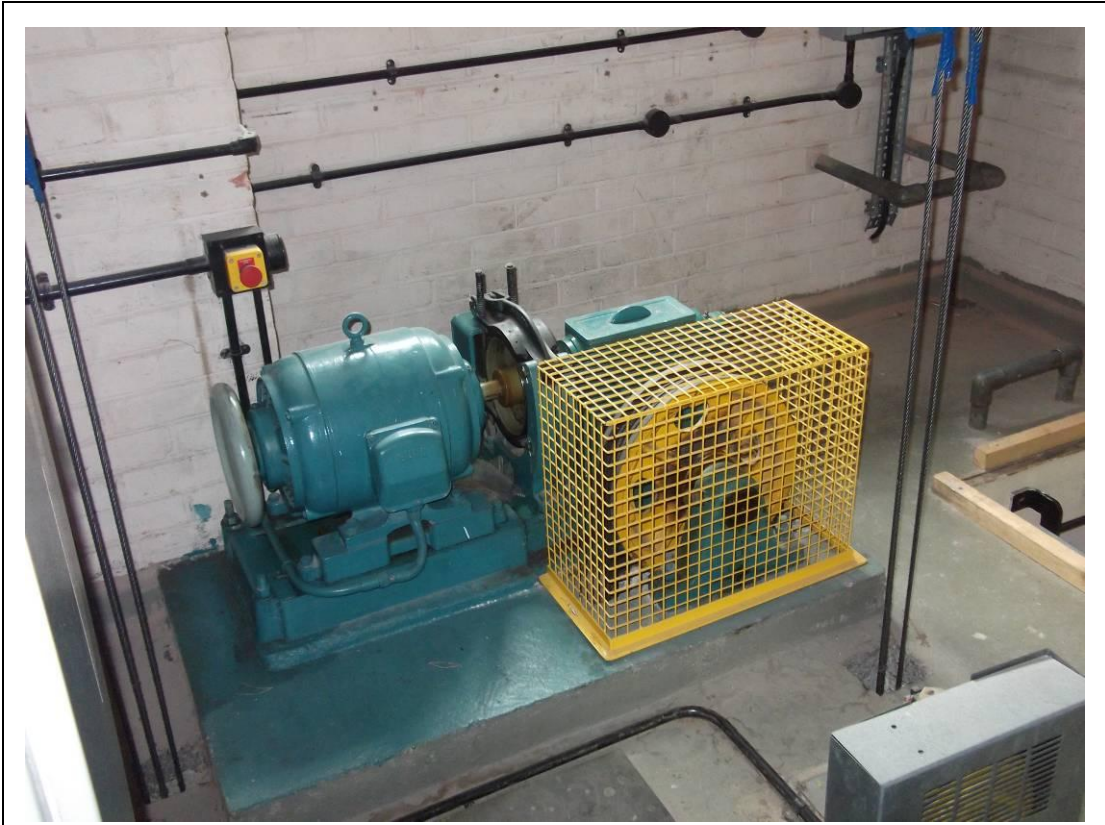
Photograph 25 (lift motor room)
