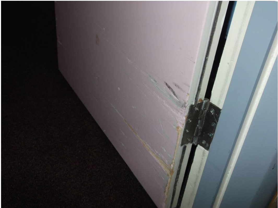
Photograph 16 (Typical damage to bedroom door)
