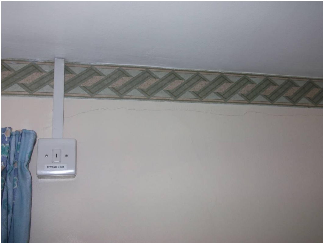
Photograph 23 (Typical cracking to plaster finish)
