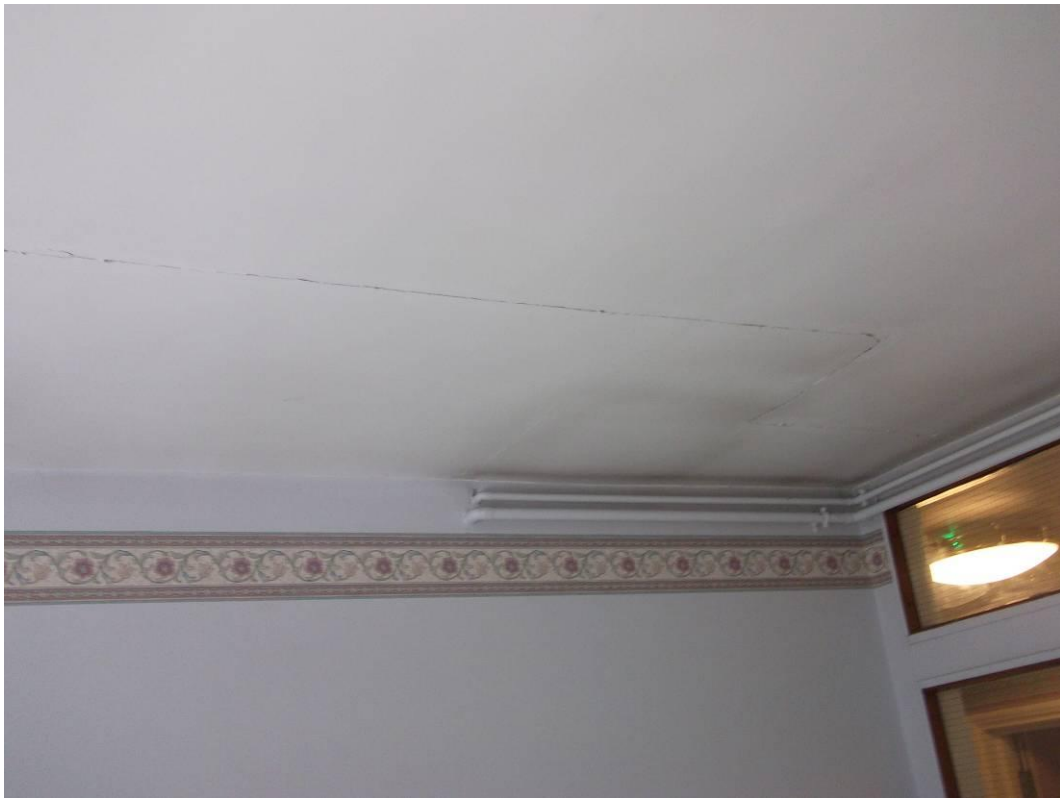
Photograph 21 (Typical plasterboard junction cracking)
