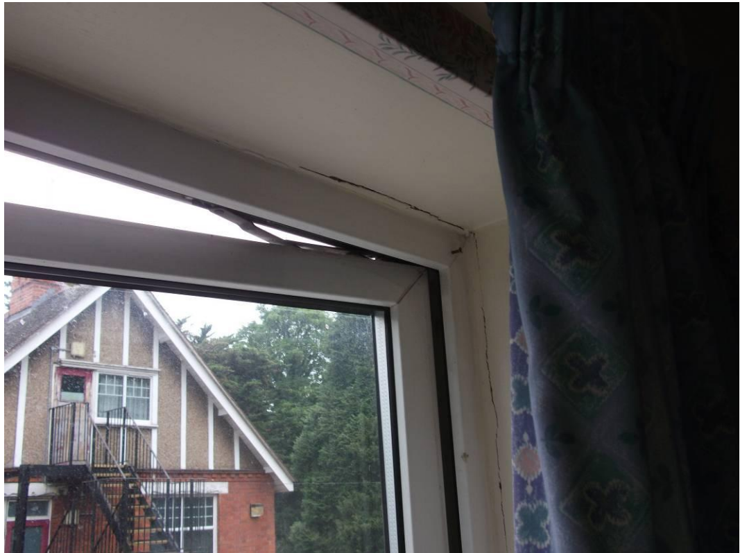
Photograph 26 (Plaster damage first floor bedroom)
