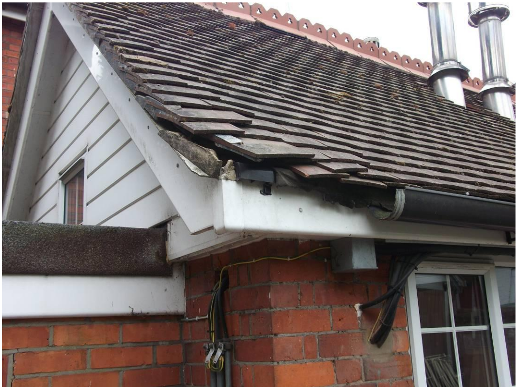
Photograph 12 (Impact damage electrical intake room)
